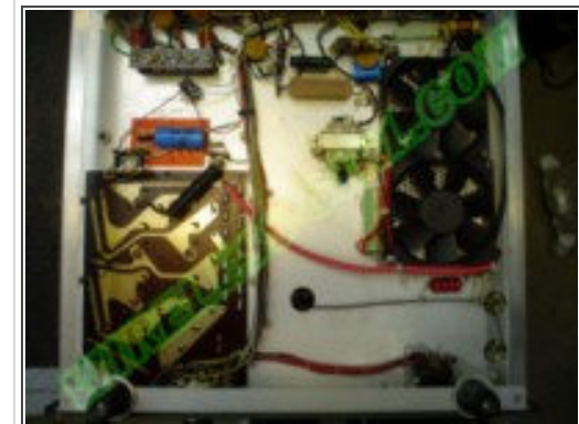
Figure 3: Bottom View Showing final wiring of the bridge rectifier and filter capacitor.
